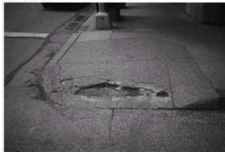
Figure 10-2. Sidewalk cracks and broken concrete are common sidewalk maintenance problems that inhibit pedestrian access to sidewalks.
